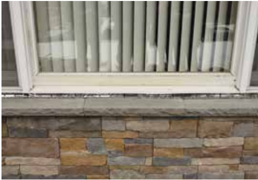
Three sills required on this window. Center and cut middle sill to avoid cut ends on end (most visible) sills.
