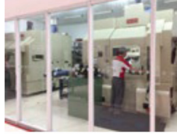
Temp. controlled "mother machine" machining room
