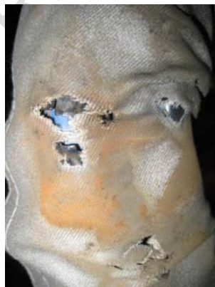
Fig. 7.2.3 (b) Damage on the cable protective sleeve
