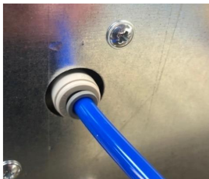
Water Connection at Boiler
