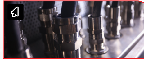
Cable Glands & Fittings
