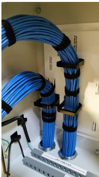
Figure 20: Copper Cable Routing showing Switch-A on the left and Switch-B cables on the right.
