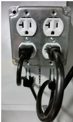
Figure 13: Outlet box and power cable secured to the back panel.
