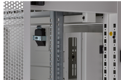
High-density vertical cable management
