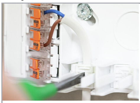
Insert the cable into the strain relief. The snap-in strain reliefs are designed for cable diameters from 4 mm to 11 mm.
