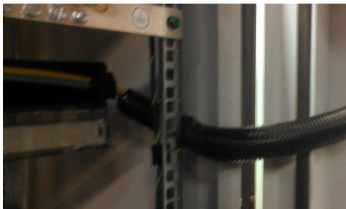
Figure 15: Loom tubing routed around hinge point and rail.
