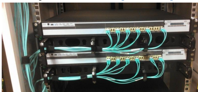
Figure 21: Fiber Switch A and B mounted to front rail showing fiber cable routing.
