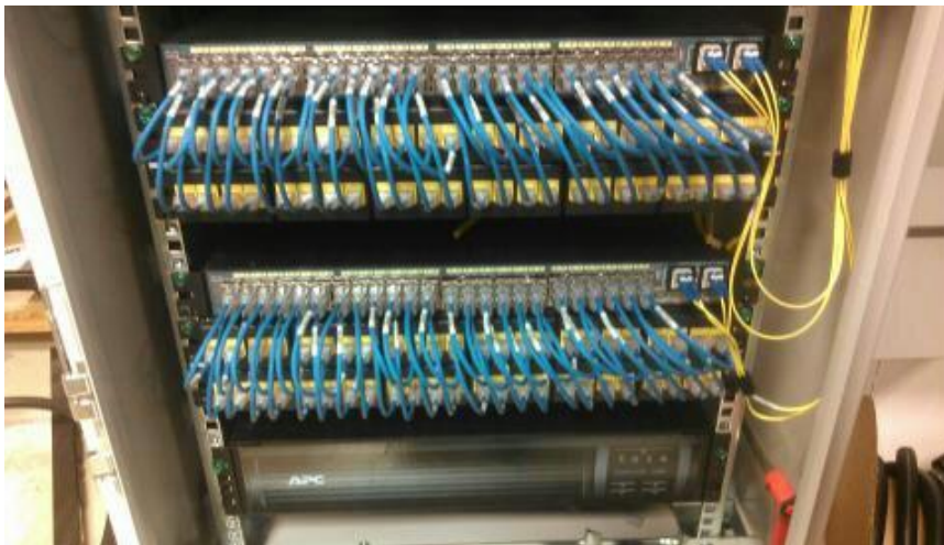
Figure 20: Switch-A (lower) and Switch-B (upper) switches showing fully populated patch cords.
