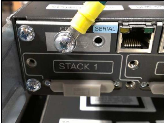
Figure 23: Ground cable connection to the Fiber switch.
