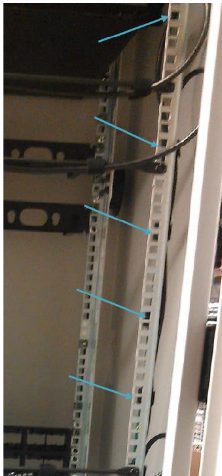
Figure 9: Fiber Power Cables A and B. View looking from the rear of the enclosure. Arrows indicate Tak-Ty locations.
