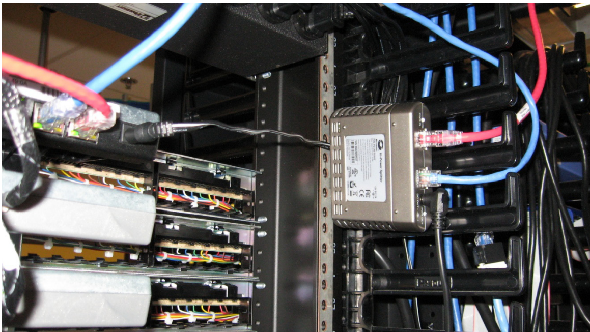
Figure E - PoE splitter mounted near Panel Manager
