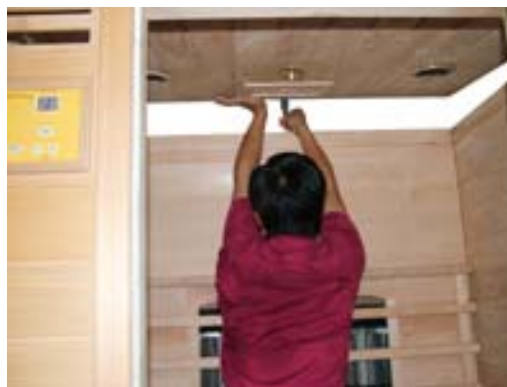
FIG-17 Leading the wires of heaters onto the board through the corresponding hole
