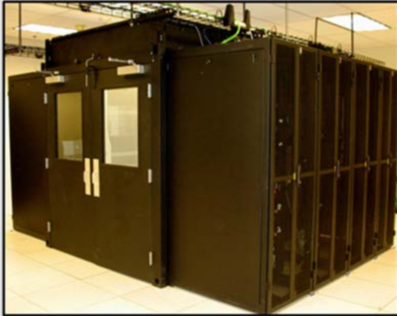
Figure 1. Cold Aisle Containment system test setup.
