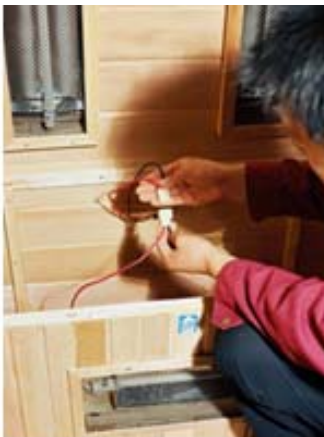
FIG-9 Connecting wire
