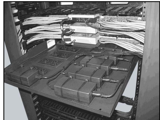
Figure 4: Rear view of rack showing power supplies placed on top of cable tie mounts and secured to shelf, which is mounted to rack from the front side.
