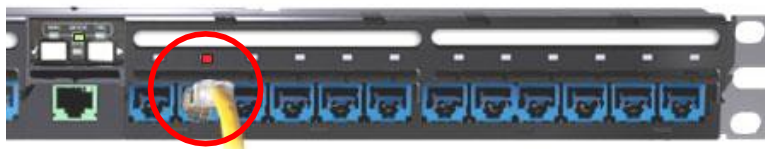
Figure 20: Secure Violation (unauthorized patch cord inserted into a port)
