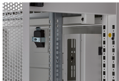
High-density vertical cable management
