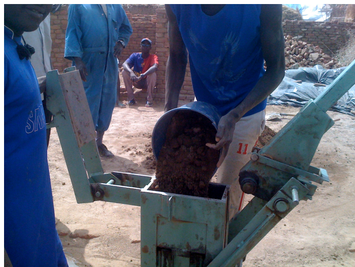
Pouring the sand, cement and water mix into the mould to make SSBs
