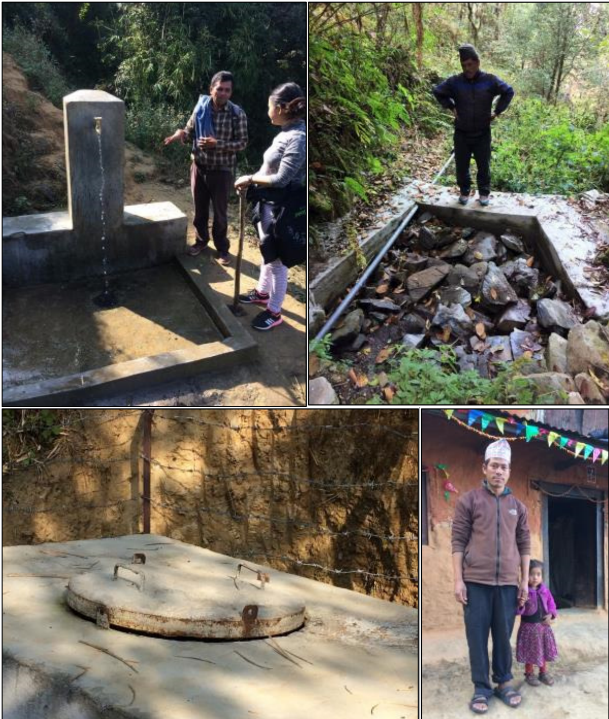
PHOTO top left: Tistung Jagdada tapstand at adult height only. PHOTO top right: Agra Chisapani GFS with no slab on the source tank. PHOTO bottom left: Agra Chisapani regulator tank with ill fitting lid. PHOTO bottom right: Rabindra Ghrung and his daughter benefit from the fresh water from Agra Chisapani GFS.
