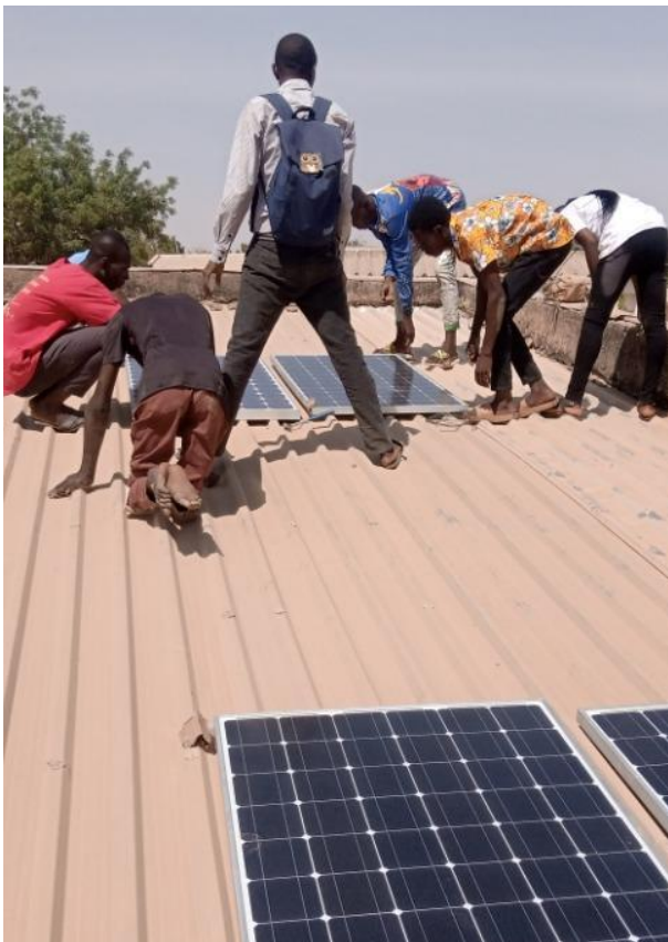
📷 Sylvestor Odey and other community members install the decentralised solar system they built on rooftops.
