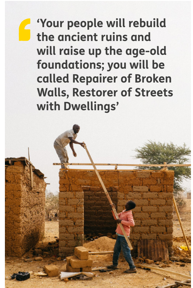
Working together to build a new home in Nigeria. Photo: Andrew Philip/Tearfund
