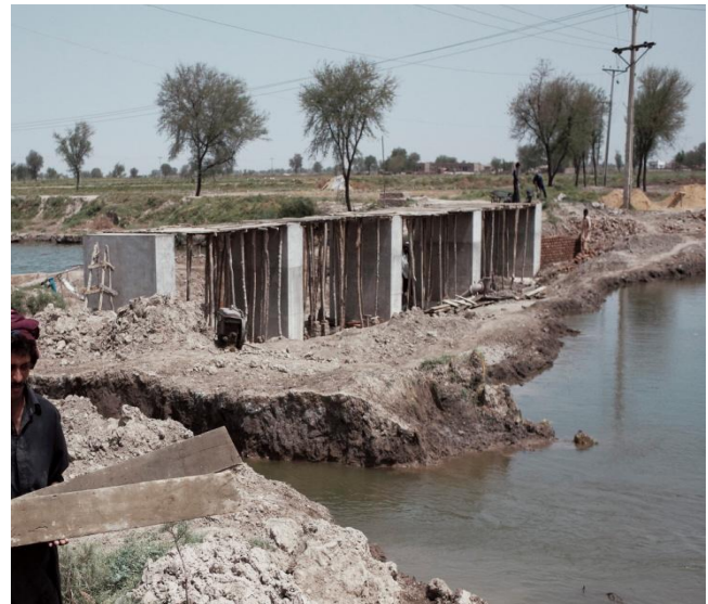
A proper bridge being built there on community request by Concern Worldwide to allow people to escape floods more easily
