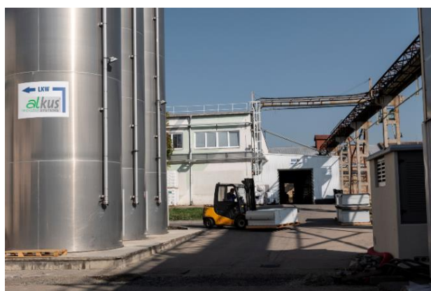
Figure 2: Polypropylene silo filling station
