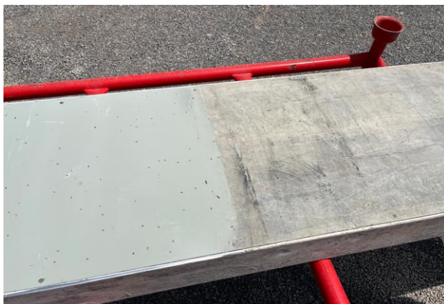
Figure 15: Frame and panel > 20 years in use (left side after repair and cleaning / right side before repair and cleaning)
