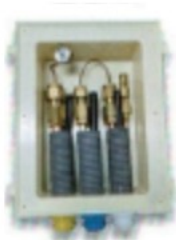
Outdoor unit room
