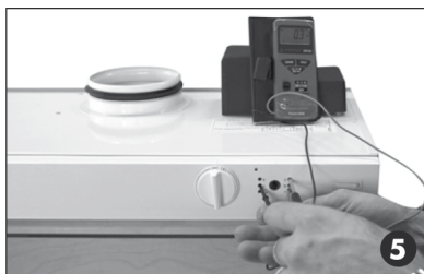
Measure voltage at contacts – and S, adjust speed 2 at potentiometer 2, and so on.
