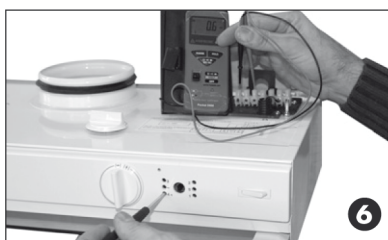
You can also carry out the measurement at the terminal block, in locations shown in the electrical diagram.
