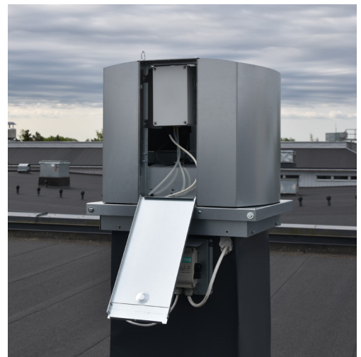
The control equipment is fully integrated inside the roof fan behind a safety door.
