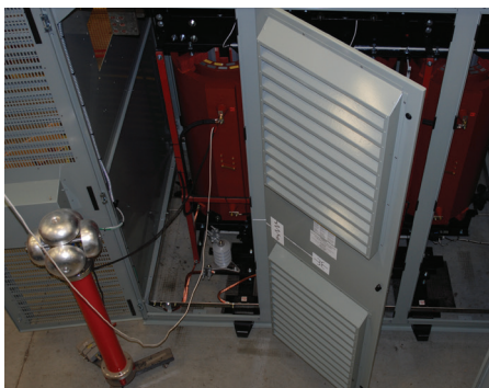
Basic Impulse Insulation Level
