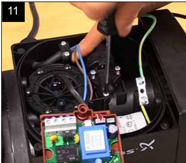
Fix the pressure switch.
