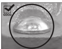
OVAL NECK OF BOLT SEATED PROPERLY
