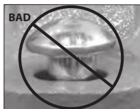
OVAL NECK OF BOLT NOT SEATED PROPERLY
