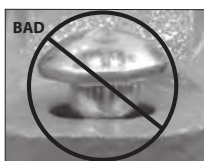
OVAL NECK OF BOLT NOT SEATED PROPERLY
