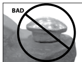
OVAL NECK OF BOLT NOT SEATED PROPERLY
