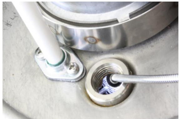
Figure 1 Gap observed by flashlight
