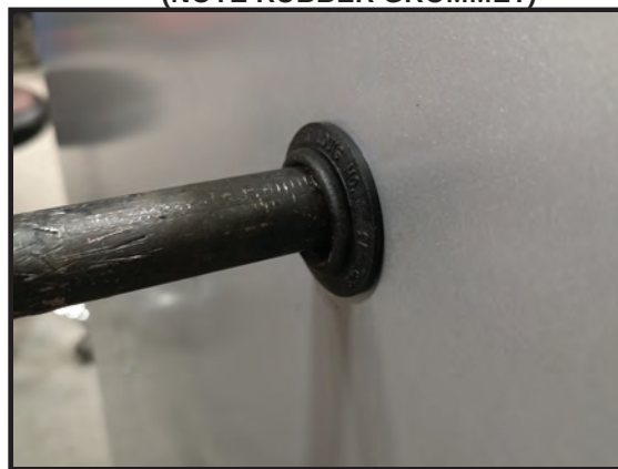
FIGURE 28 - FURNACE GAS PIPE CONNECTIONS (NOTE RUBBER GROMMET)
